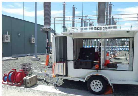
Purpose built trailer carrying 8kVA Earth system
